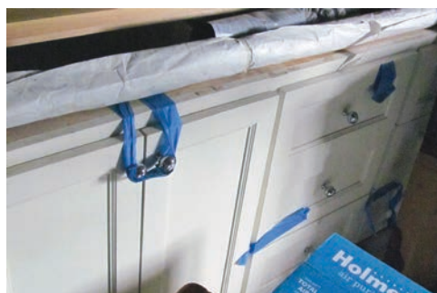
The cabinet set Justine found at the Reuse Center is awaiting installation. The set was just what she was looking for, at a fraction of the cheapest new cabinet set she could find.
