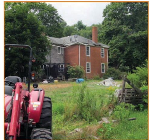
This historic home had fallen into major disrepair before Justine purchased it. One step at a time, she is restoring it to its former beauty.
